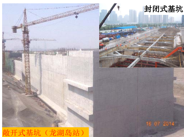
Figure 9. Form of foundation pit of Longhu Island Station 图9. 龙湖岛站基坑形式
