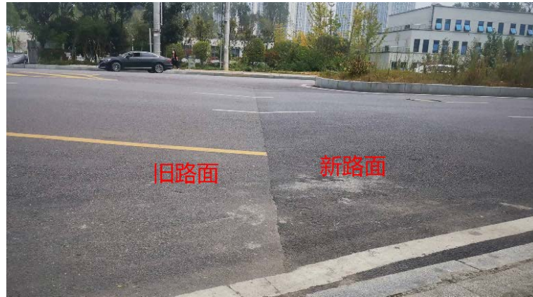
Figure 2. The junction between old and new roads is not smoothly connected on site
