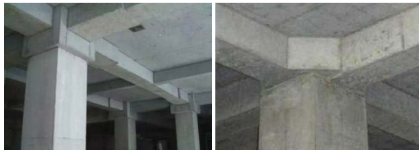
Figure 3. Strengthen the core region of concrete beam-column joints by enlarging the section
