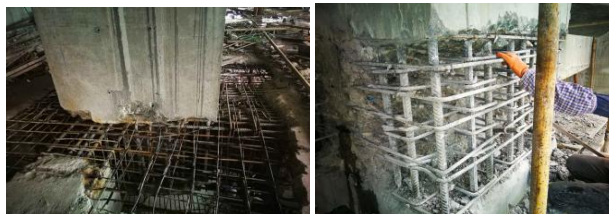
Figure 7. Appearance of chiseling construction completed in the core region of some side column-beam joints on the first floor
