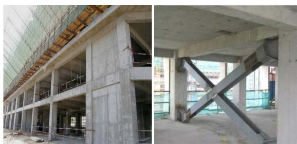
Figure 6. Strengthen the core region of beam-column joints by adding shear wall or support between columns
