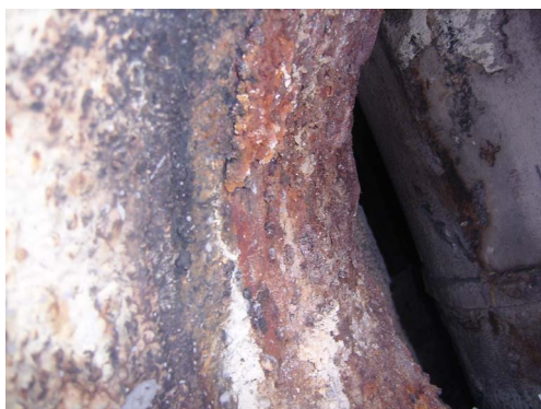
Figure 1. Localized corrosion photo of desulfurizing tower 图 1. 脱硫塔局部腐蚀照片
