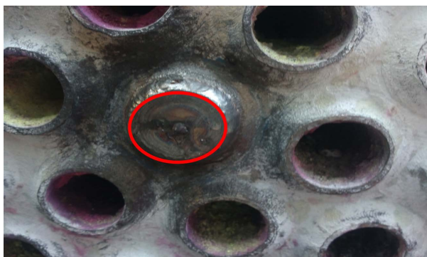
Figure 5. After repairing the end tube plate of a cold and rear end bundle
