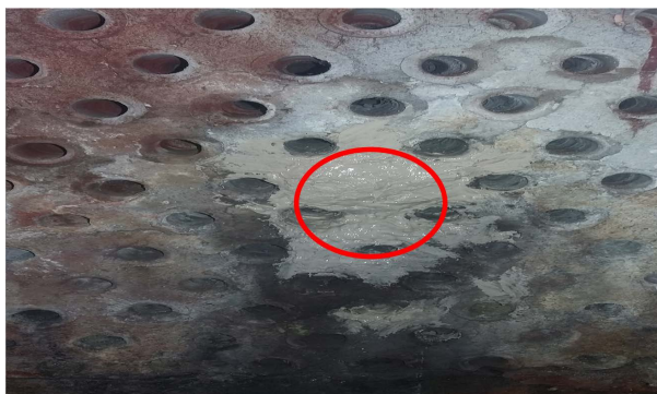
Figure 4. After repairing the end tube plate of a cold front and rear bundle
