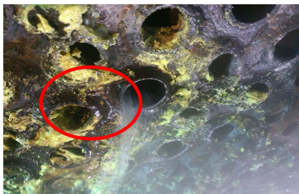
Figure 3. 1 leakage of cold and end tube bundle 图 3. 一冷后端管束泄漏
