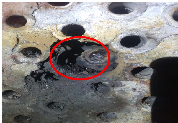
Figure 2. 1 leakage of cold and front tube bundle 图 2. 一冷前端管束泄漏
