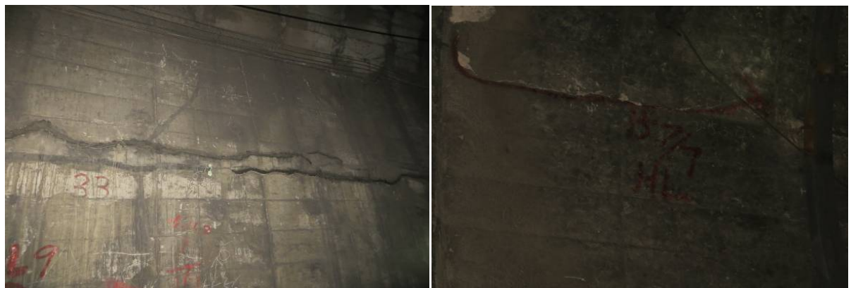
Figure 3. The situation of the outer drum of the tunnel cracking 图 3. 隧道开裂外鼓情况图
