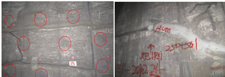
Figure 5. Sidewall anchor rod and grouting remediation measures 图 5. 边墙锚杆和注浆整治措施
