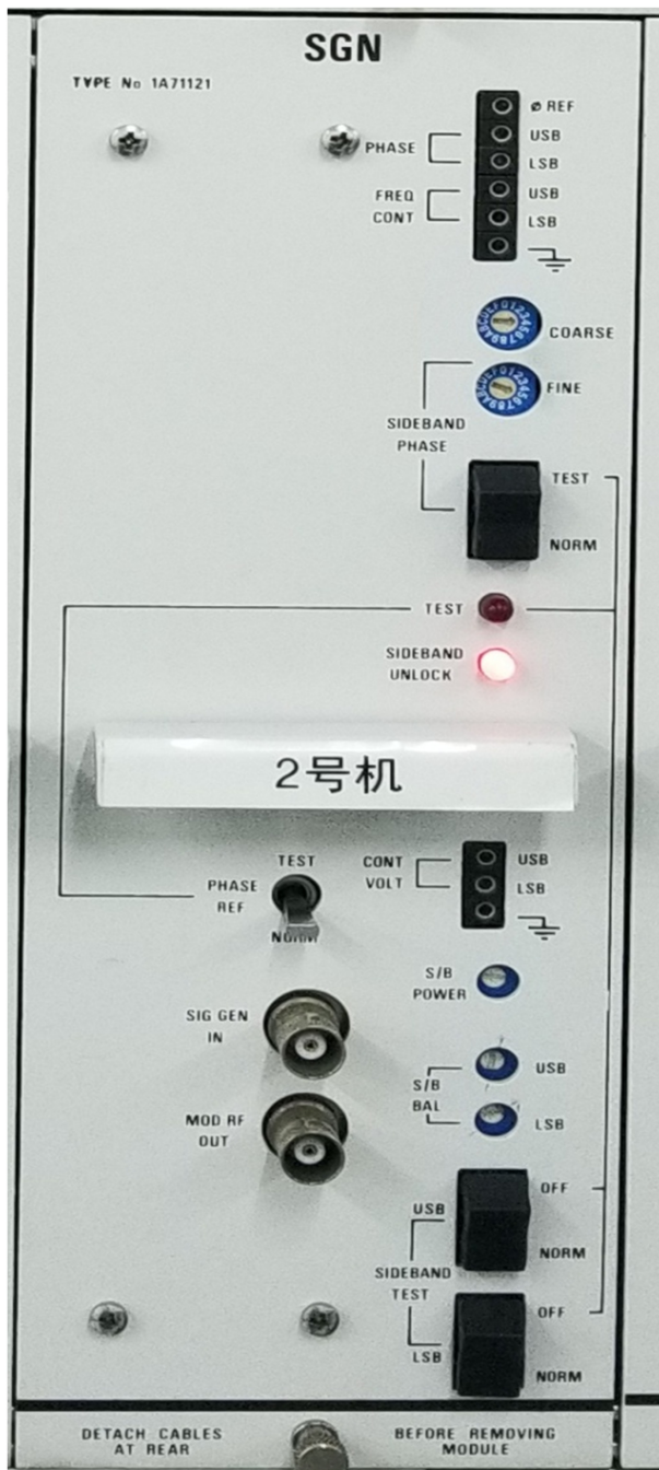
Figure 2. The second fault phenomena 图 2. 设备故障现象二
