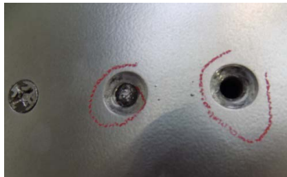
Figure 2. Rivets come off and paint is bulging 图 2. 铆钉脱落以及漆层鼓包
