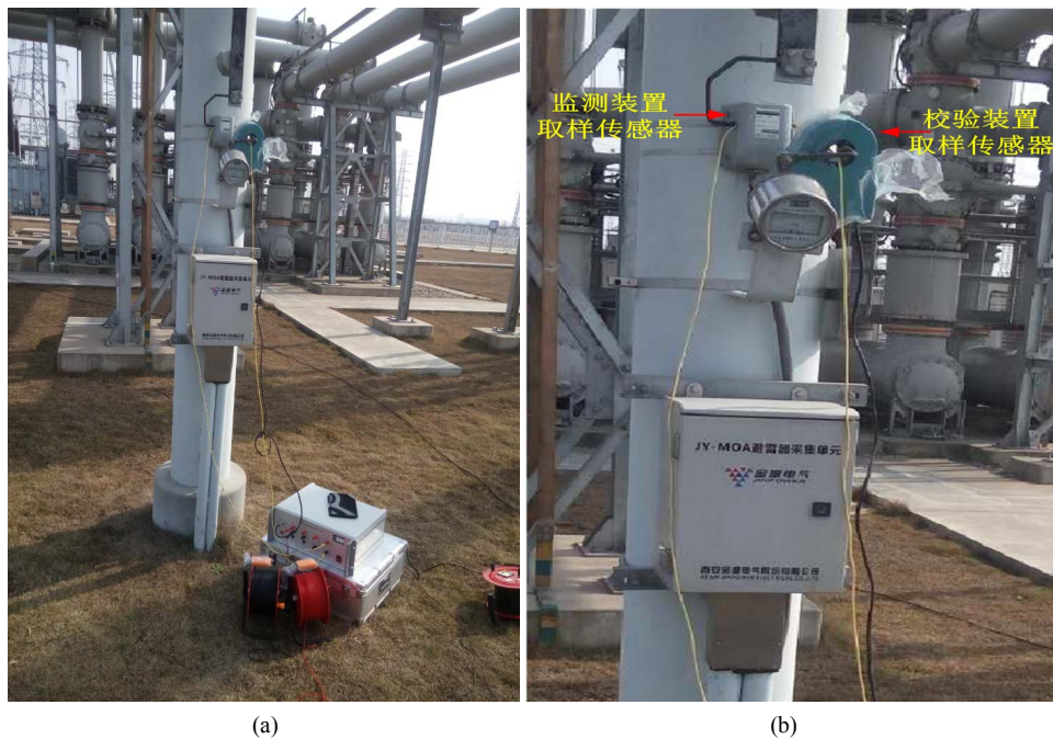
Figure 8. Field verification; (a) the platform of verification; (b) MOA linkage current transducer 图 8. 现场校验图; (a) 校验平台搭建; (b) MOA 在线监测传感器
