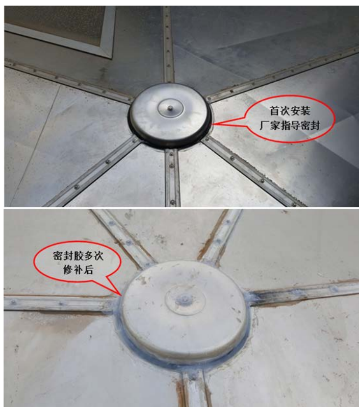
Figure 1. Before and after repairing 图 1. 修补前与修补后对比
