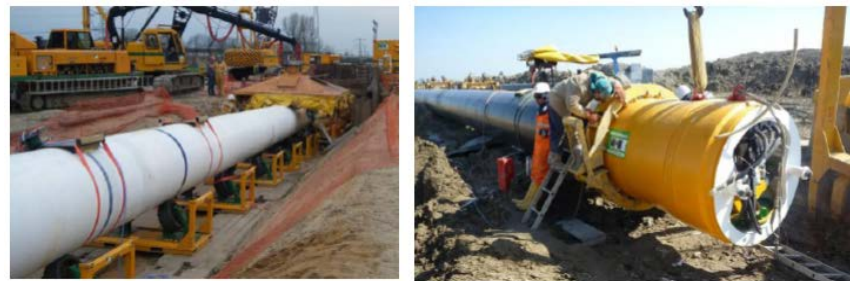
Figure 13. Installation for the fourth part of the pipe thrusting unit 图 13. 第四节主机安装
