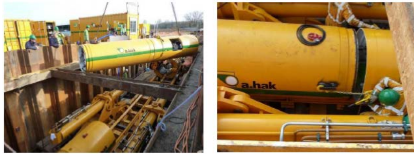
Figure 12. Installation for the first three parts of the pipe thrusting unit 图 12. 前三节主机安装
