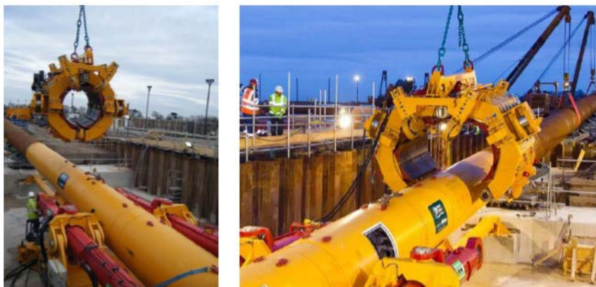
Figure 16. Installation of the clamping unit on the pipeline 图 16. 管道夹紧器安装
