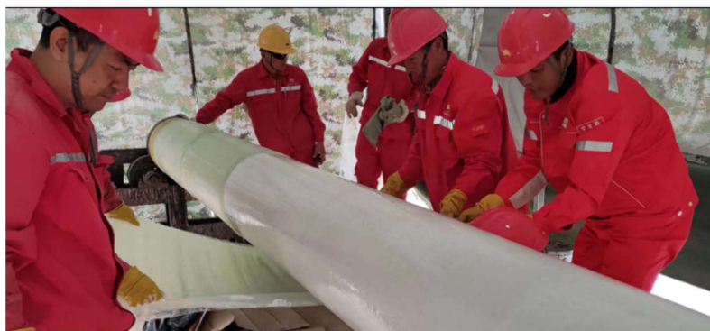
Figure 1. CND400 photosensitive curing FRP prepreg tape coating construction 图 1. CND400 光敏固化玻璃钢预浸带包覆施工
