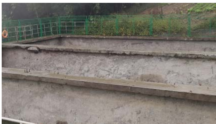
Figure 3. Damage status of a shale gas pool 图3. 某页岩气水池损伤现状
