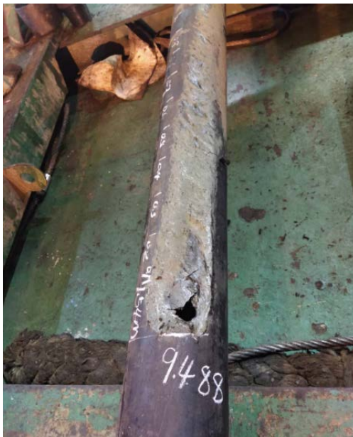
Figure 4. Cut out damaged casing 图 4. 切割出破损套管
