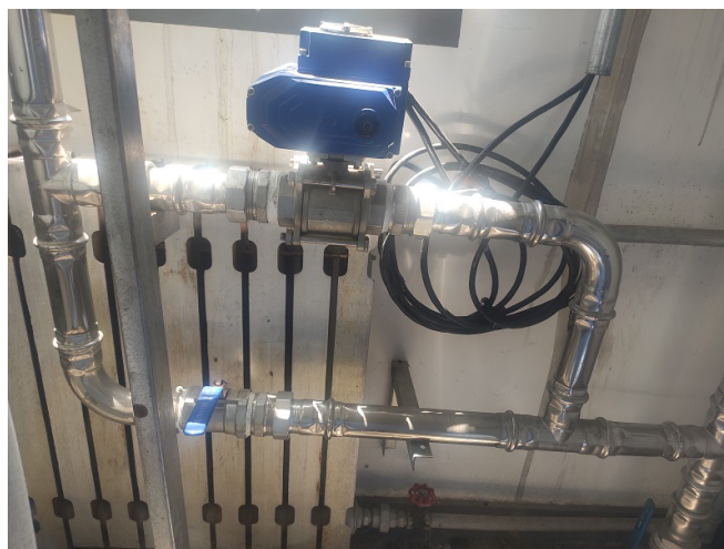
Figure 4. Water make-up valve of pool 图 4. 水池补水阀
