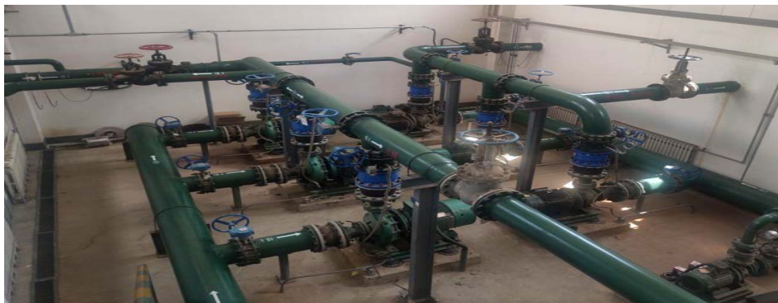
Figure 1. Main equipment of cooling circulating water system
