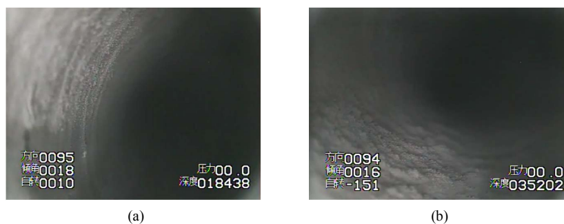
Figure 4. 2# borehole TV camera. (a) 2# is not affected by mining area (18.4 m); (b) 2# affected by mining area (35.2 m)
