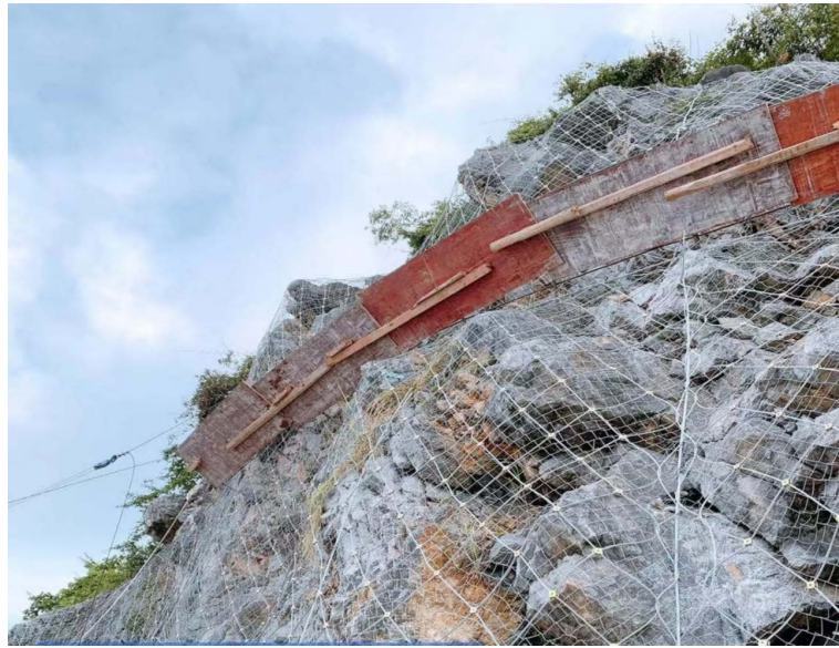
Figure 2. Dangerous rock active protection net 图 2. 危岩主动防护网
