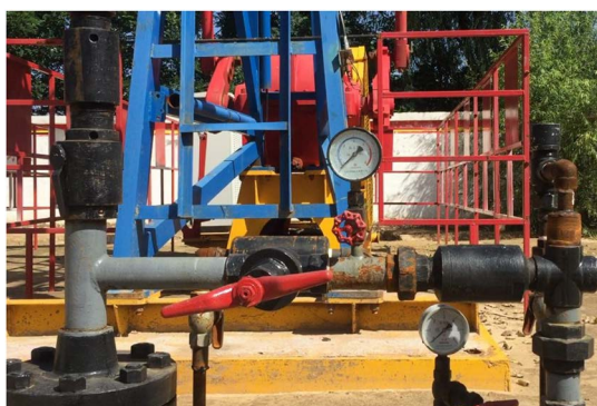
Figure 2. The wellhead pressure decreases during down stroke operation of pumping unit 图 2. 抽油机下冲程运行井口压力降低
