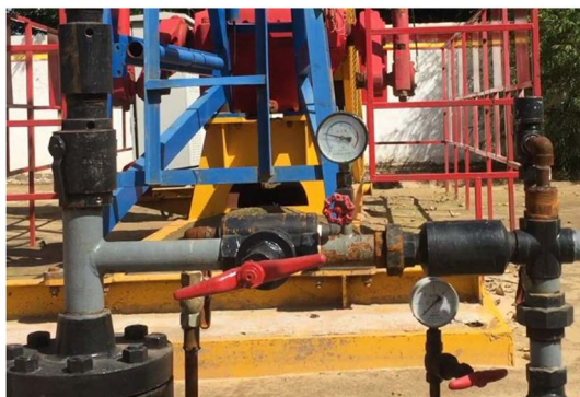
Figure 3. The wellhead pressure increases during the upper stroke of pumping unit 图 3. 抽油机上冲程运行井口压力升高
