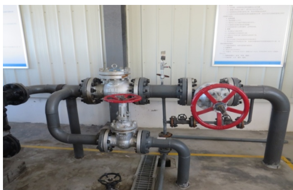
Figure 2. Pipeline at pump outlet
