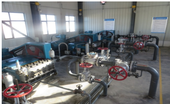
Figure 1. The export pump of JD central process facilities
