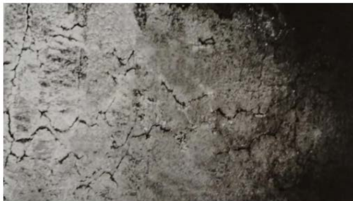
Figure 6. Macroscopic characteristics of steel plate crack
