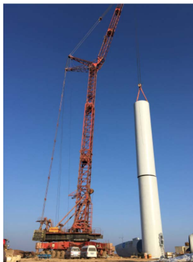
Figure 1. Hoisting machinery of fan
