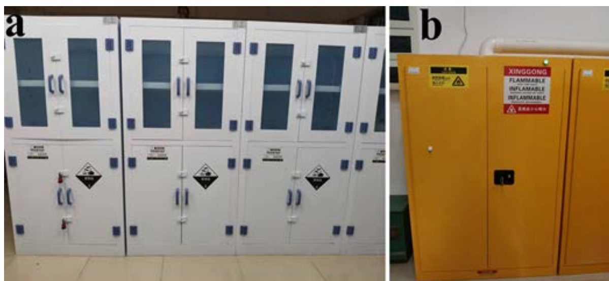
Figure 1. (a) Acid-base cabinets and (b) explosion-proof cabinets are used to store drugs on this floor
