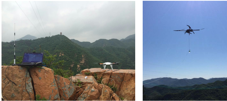
Figure 6. Application of UAV in line construction of mountain area 图 6. 山区线路工程施工无人机放线应用
