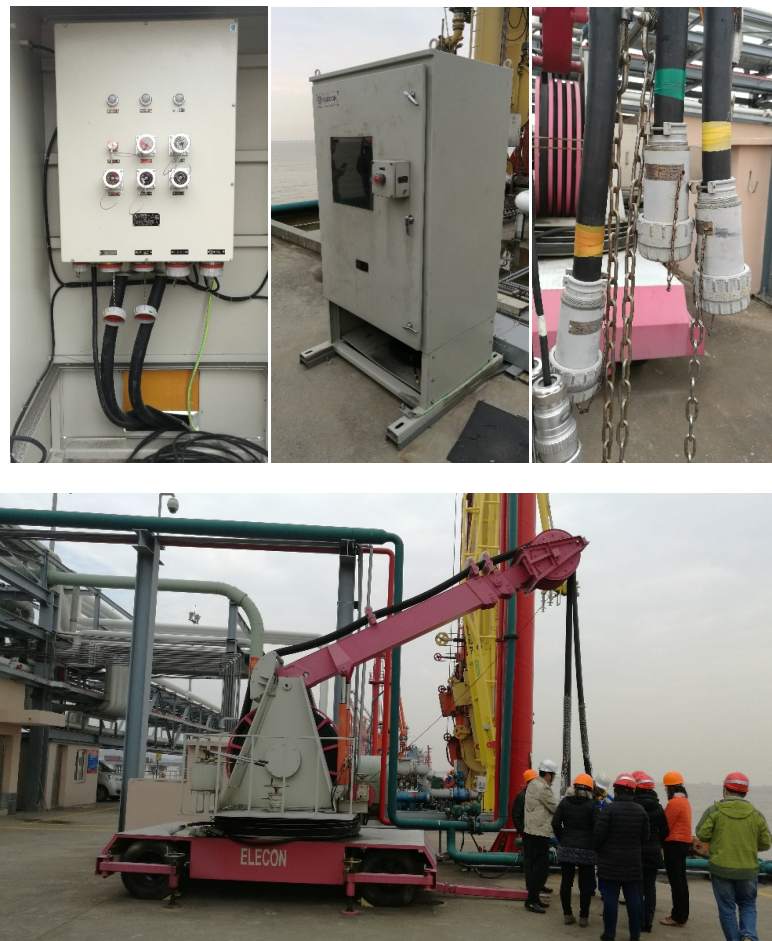
Figure 6. Shore power facilities of Jiagang Petrochemical Wharf 图6. 嘉港石化码头岸电设施
