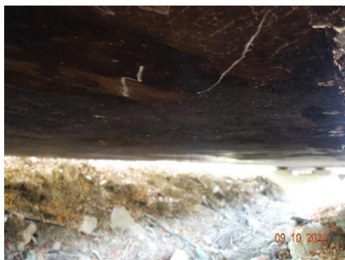
Figure 2. Floor blackened, concrete spalling 图 2. 底板熏黑、混凝土剥落
