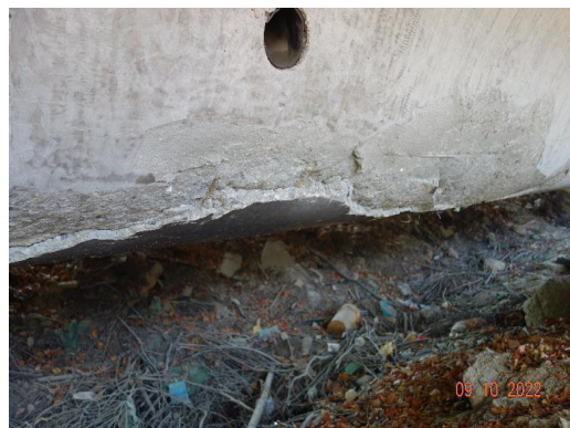
Figure 1. Web concrete spalling, steel bar exposed
