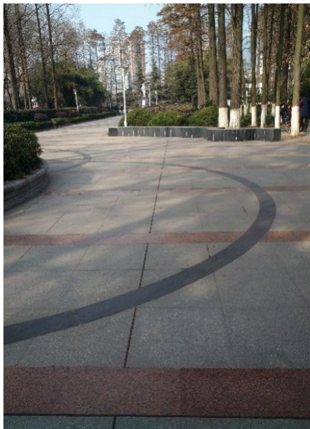
Figure 8. Cool-colored pavement in a circular square
