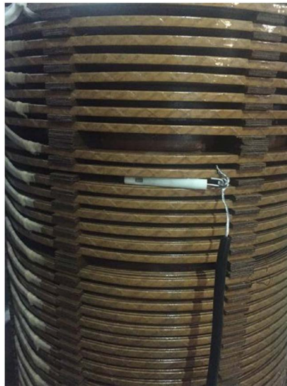
Figure 17. Placement of partial discharge power supply in low voltage winding 图 17. 局部放电源在低压绕组的放置方式
