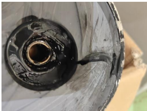
Figure 31. 35 kV Electric power cable express the connect point
