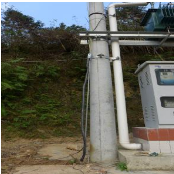
Figure 2. Flexible graphite composite grounding material and the original network connection 图 2. 柔性石墨复合接地材料与原地网的连接
