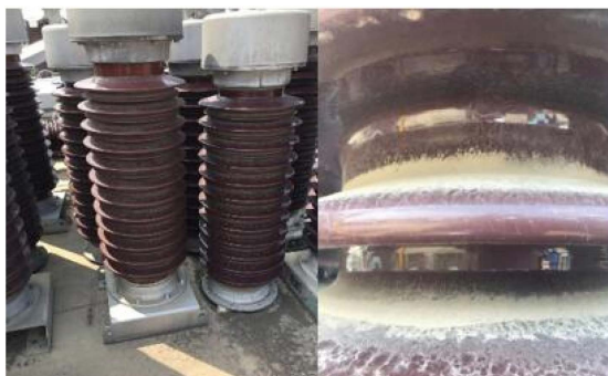
Figure 1. Insulators to be cleaned
