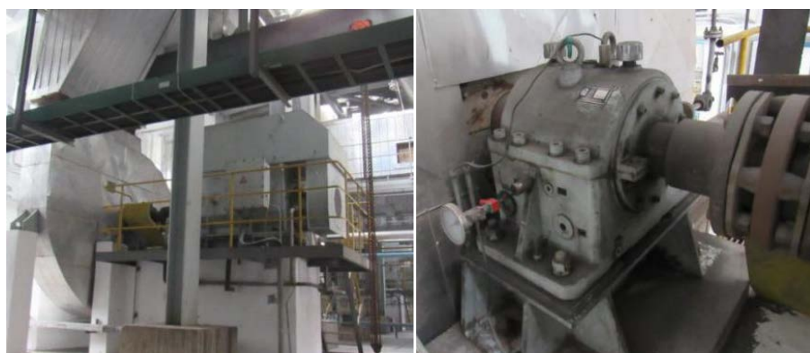
Figure 2. Explanation of the functions of the primary and secondary fan bearing seats in a circulating fluidized bed boiler
