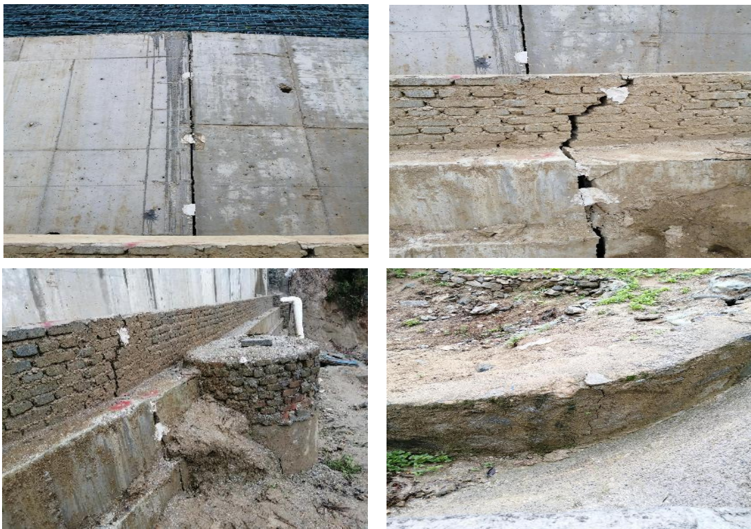
Figure 4. Crack in the right side of the slope 图 4. 边坡右侧挡墙裂缝
