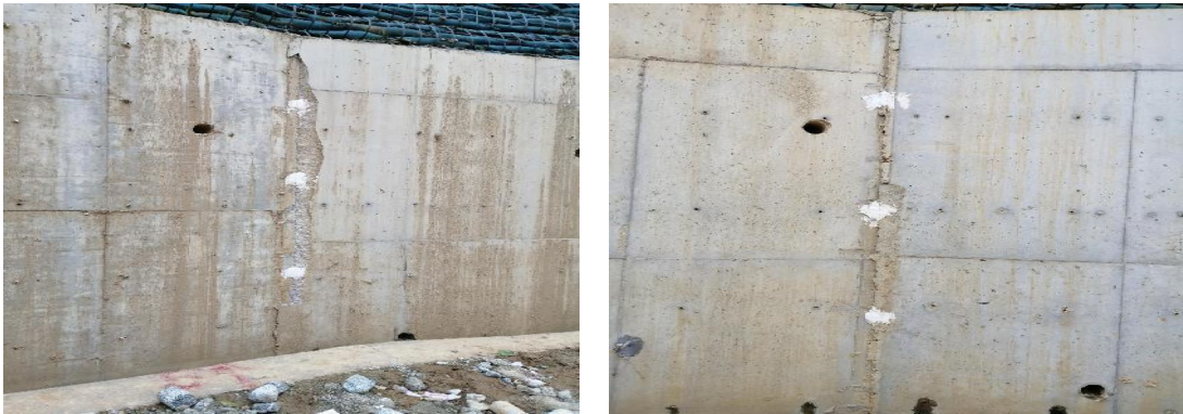
Figure 3. Cracks in the middle retaining wall of the slope 图 3. 边坡中部挡墙裂缝
